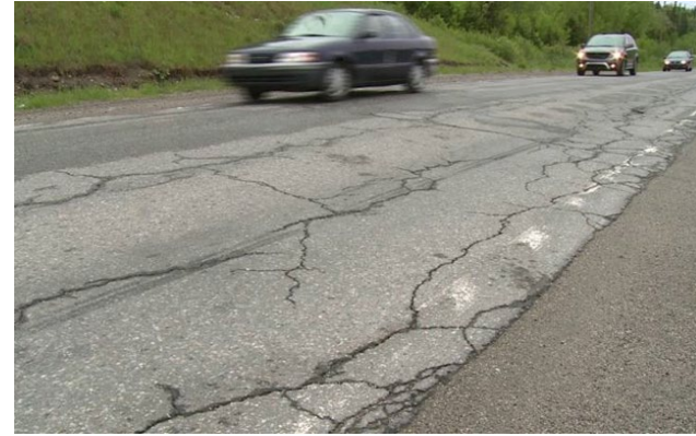
도로품질 저하 (Road deterioration)
